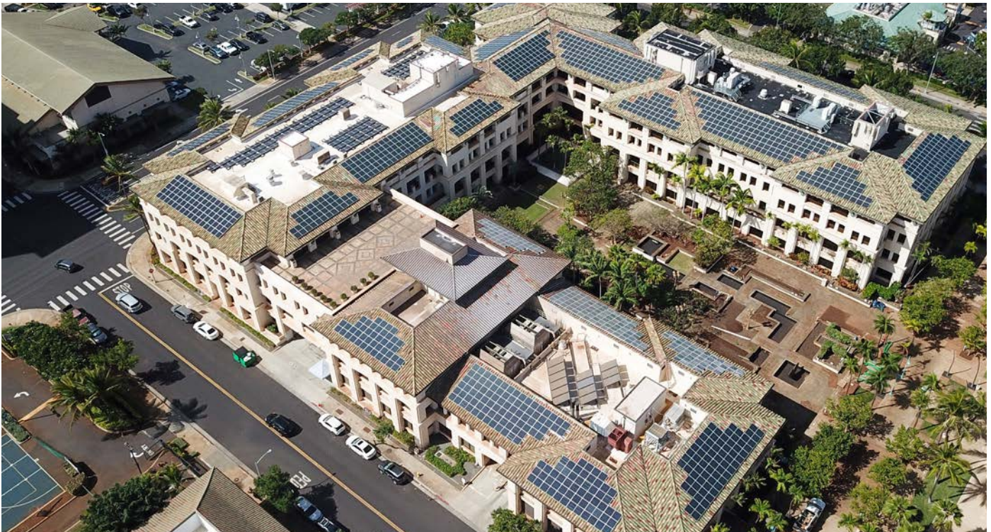
Bank of Hawai'i has installed photovoltaic solar panels on over 60% of owned branches and buildings, including its Hale O Kapolei facility (pictured above).
